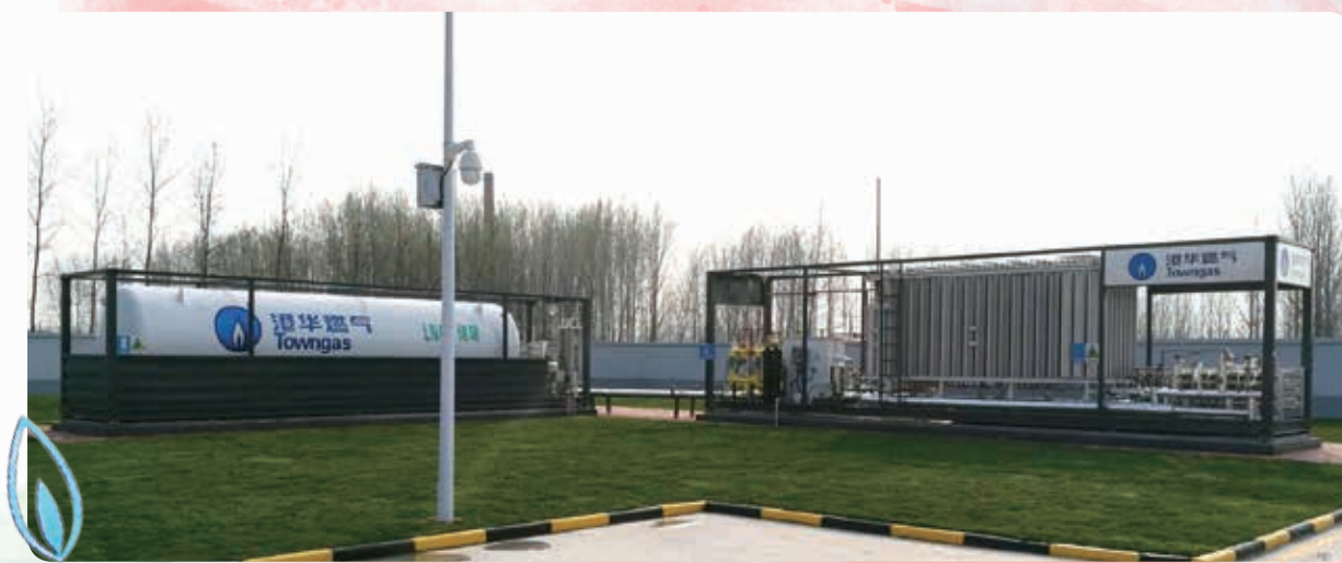
This innovative skid-mounted small liquefied natural gas transition station was developed and designed by our Engineering Department. We have obtained a national invention patent and three utility model patents for the design.
